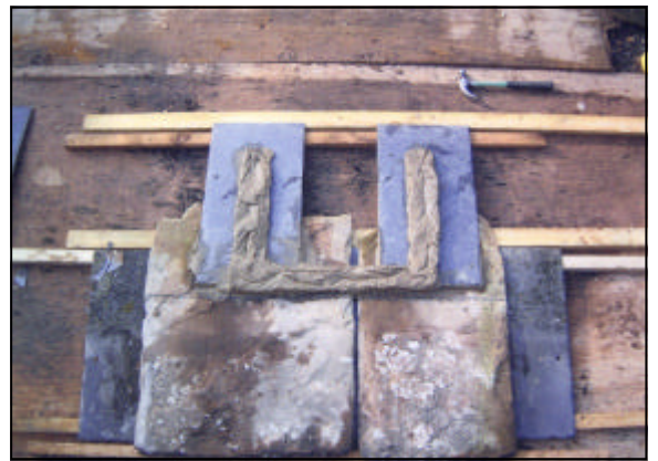
Figure 7 Mortar bed placed to receive the stone-slate. These shadows are 300 mm wide.
