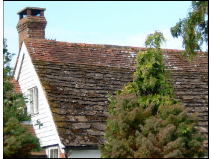
Figure 11 It is quite common nationally for stone slate to have been replaced with some other locally traditional material such as clay tiles. This is recognised as a traditional technique and should be conserved.
