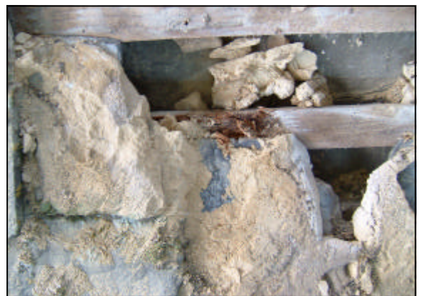
Figure 9 If the bedding mortar reaches the battens moisture will be drawn to them causing rotting.
