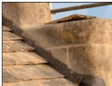
Figure 16 Mortar fillets are particularly prone to cracking due to differential movement between the wall and the roof. This can be prevented by separating them from the roof surface and reinforcing them with stainless steel expanded metal
