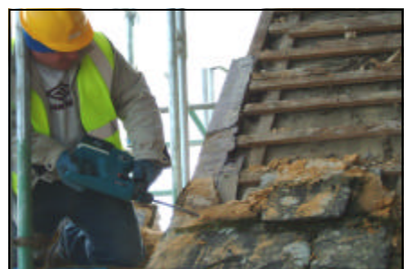
Figure 19 Bedding mortar must not be so hard or so adhesive that it damages the stone-slates when it eventually needs to be removed to relay the roof. Hard mortar being removed with a jack hammer.
