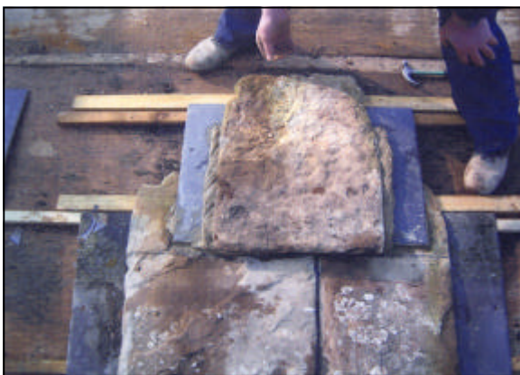
Figure 8 Stone-slate in place. Note how the vertical mortar beds do not reach the batten where they would cause rotting.
