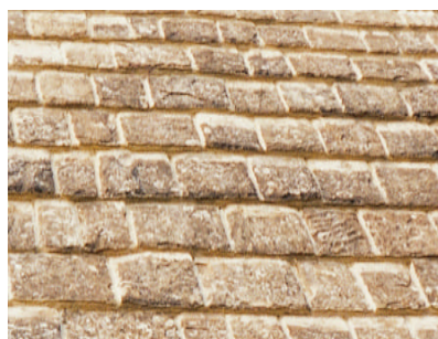
Figure 24 The mortar in the perpendicular joints and under the tail of the stone-slates should be raked out rather than left showing as here.
