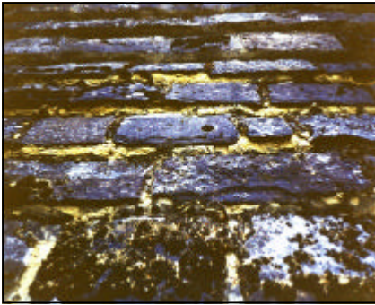
Figure 20 Single lap Horsham roofs rely on the mortar to be weather-tight. To avoid failures such as the disintegration of a weak mortar as shown here it is essential to ensure the correct constituents are accurately measured and carefully mixed.
