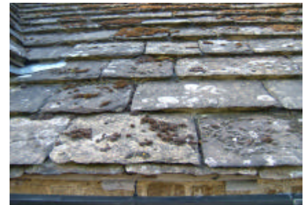
Figure 1 Horsham stone-slates or flags are calcareous, flaggy sandstones. 'Nowhurst has been quarried for several hundreds of years but the roofing stone comes in patches. We find a stratum about three feet down with now and again a hard patch in it. This stratum varies in depth from two feet to five feet and it is from this that the roofing stone comes. The base of the stone is sandstone but for some reason there is lime in the roofing stone patches which hardens it into a granity stone. You can't split any stone for roofing. The natural cleave has to be there. If the stone has a tight cleave we let it stand in the wind and frost for some months, and the weather helps to split it perfectly.' (Dunkerton, F. J. 1945, Quarry Manager's Journal, p213)
