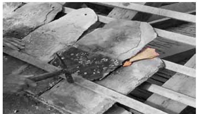
Shale Example in Collyweston slating used to support the slate above and pointing any penetrating water onto the slate below
