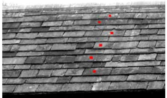
Pigs Incorrect gauging in a Carboniferous sandstone roof
