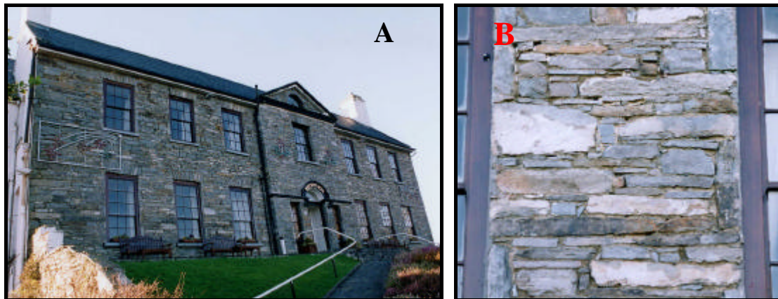
Figure 6: A & B. View of the circa 1760 Ennistymon House (the present Falls Hotel). Render has been removed revealing the roughly coursed rubble walls constructed with the local sandstone.
