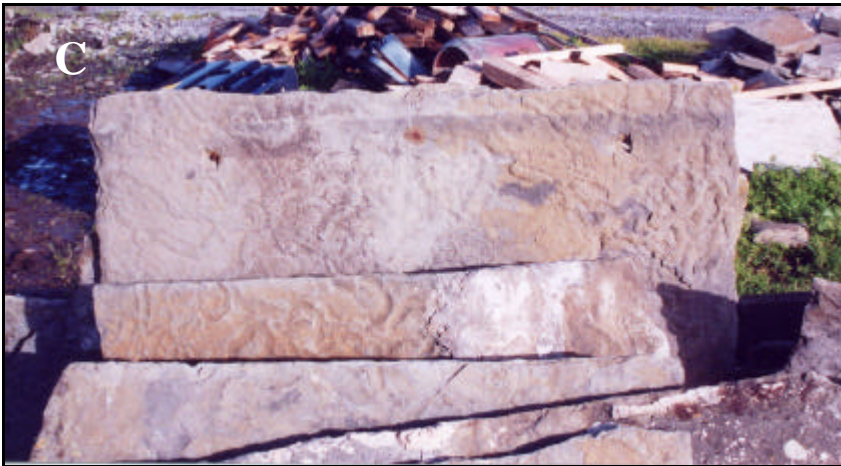
Figure 11: Figures A-C show stone slates after removal from roof. Note holes for nails in flag head below & the distinctive fossilized trails of the Moher slate.
